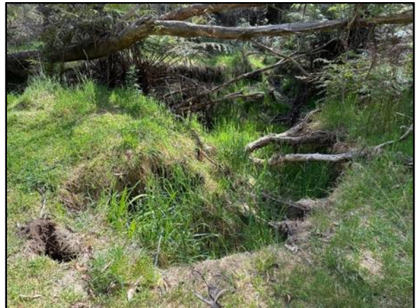
Stormwater from Gordon Road is causing major damage in the national park.
