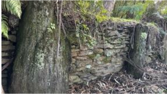
Dry-stone retaining walls in poor condition
