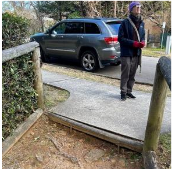
Unsafe entrance to park
